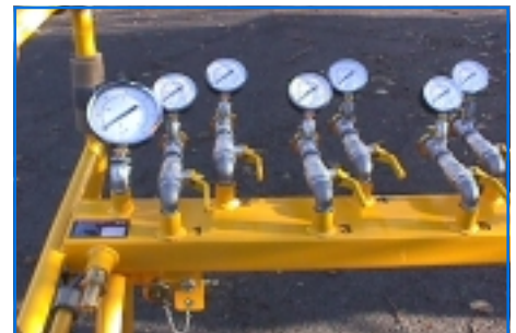
Control Valves and Pressure Gauges on Console 10001-20
